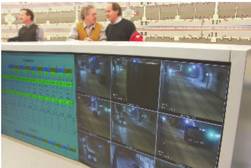
Tunnel Control Centre – the focus point in an emergency
