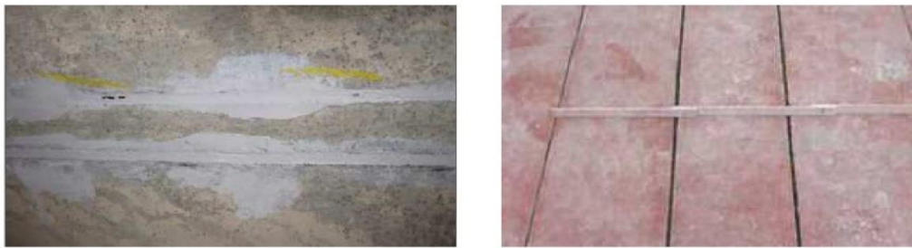
Fig. 6. Reinforcement installed in slots with CFRP lamellae on the underside of a cross-section (left) and slots prepared for installation (right), taken from [16].
