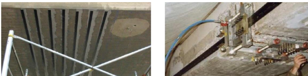
Fig. 5. Bonded CFRP laminations on the underside of a cross-section (left) and prestressing of CFRP laminations (right), taken from [16]
