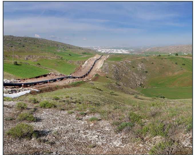
Figure 4: TANAP is passing on the upper side of a large solution doline
