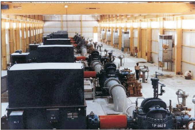
Abb. 6 Pumpstation des Riyadh Water Transmission Systems
