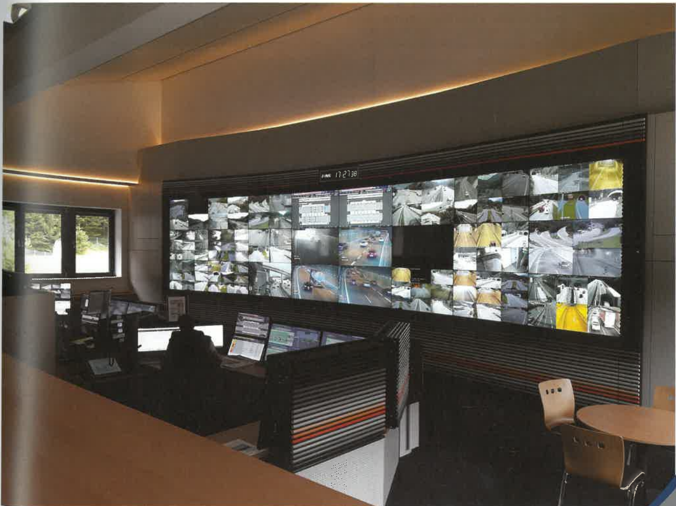
Illustration 3 - A modern control centre at Arlberg Tunnel (Austria) – The brain behind operational measures © ASFINAG
