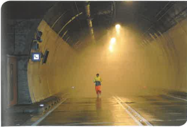
Illustration 4 - Fixed fire fighting system in operation - Bregenz City Tunnel (Austria) © BAST
